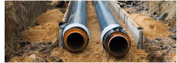
Installation constraints and pipework
